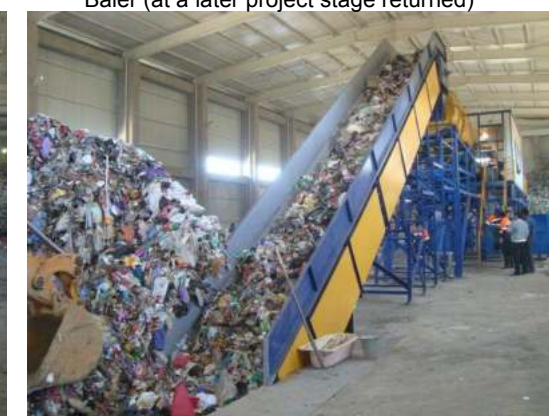
Waste feeder in operation
